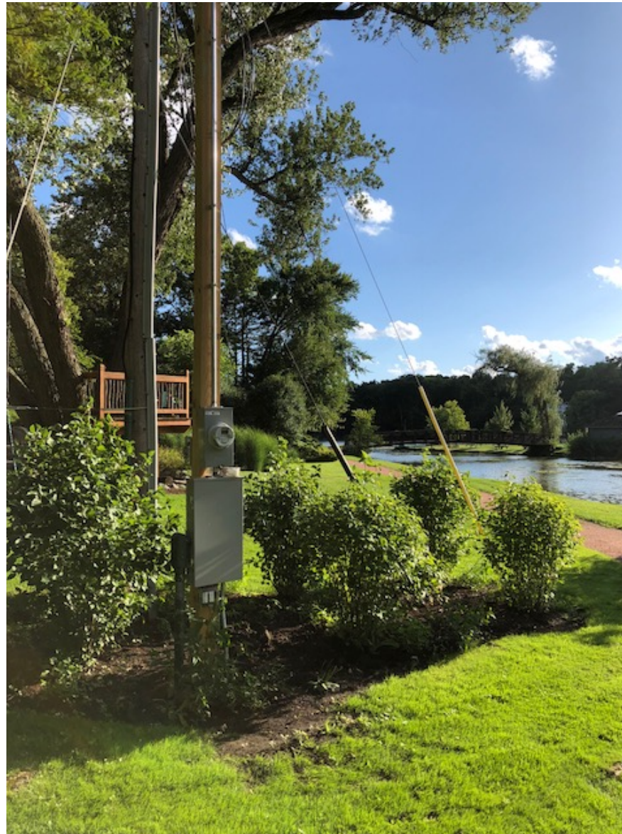
New electric pole and upgraded electric service to Rest and Toy Island Now up to code.
