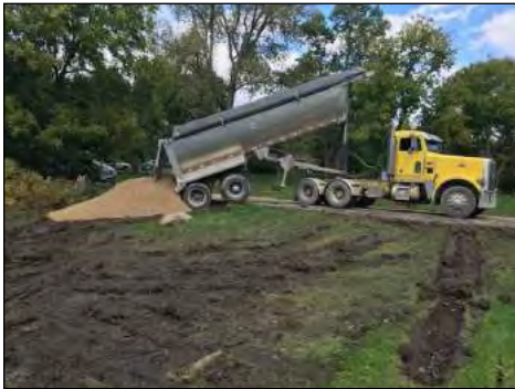
The first of 3 loads of material gets dropped at the SE boat landing
